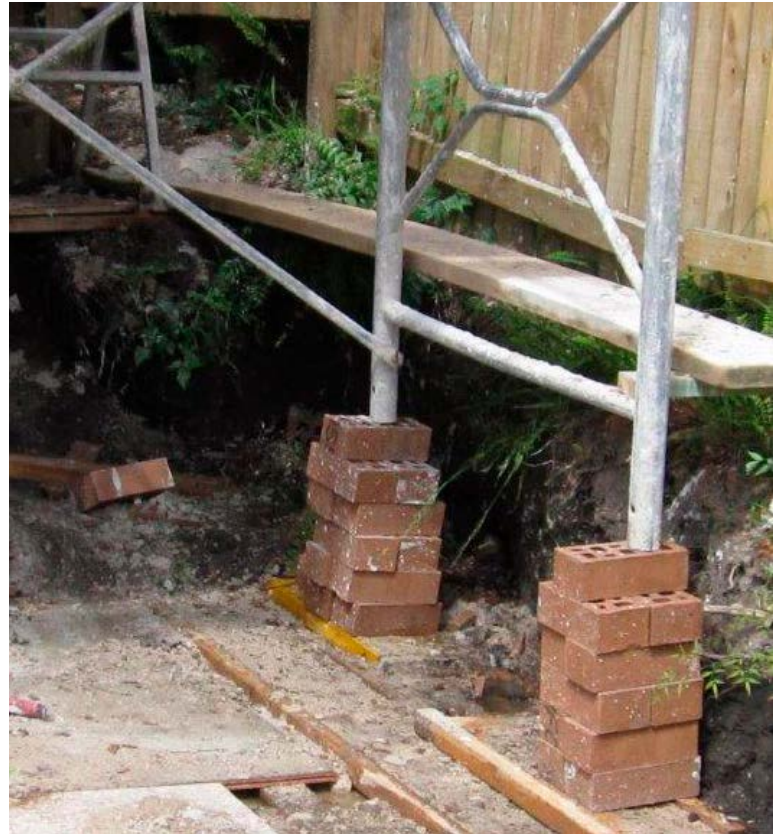
Picture 2: Scaffold on an unstable foundation.
