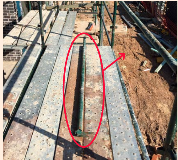
Picture 4: Scaffold with mid rail removed.
