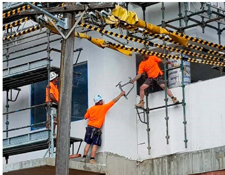
Picture 3: Workers accessing incomplete scaffold and misusing it.
