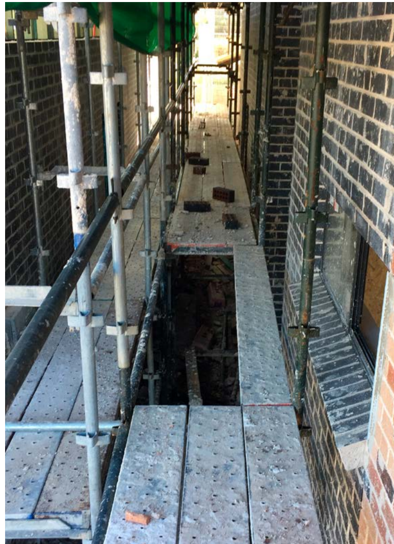
Picture 1: Scaffold with missing planks
