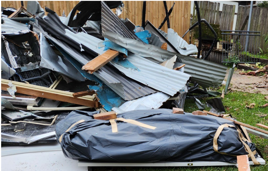
Photo 2: Example of asbestos waste “parcel” not suitably sealed, contained and secured in a manner that facilitates its future safe disposal
