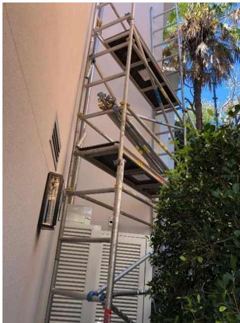
The scaffold structure on the site of the incident
